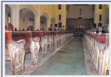
Pictured is the water level inside the church sanctuary following the hurricane.
